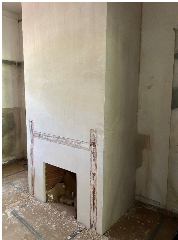
New fireplace in 48 East Lawn, approximately where the arch is in the photo on the left
